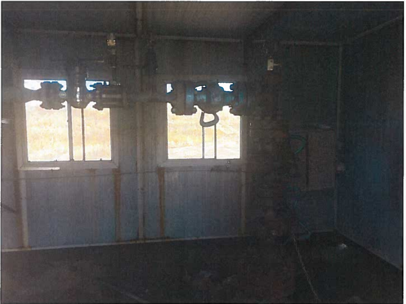
Photo # 1: Well head located inside building
