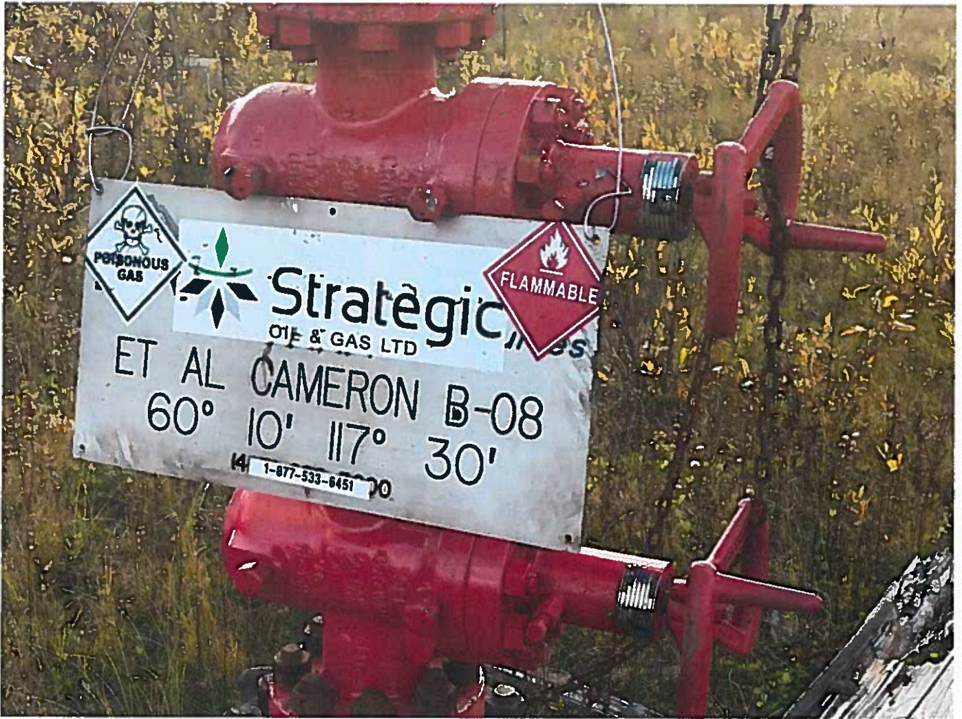
Photo # 1: Well head
