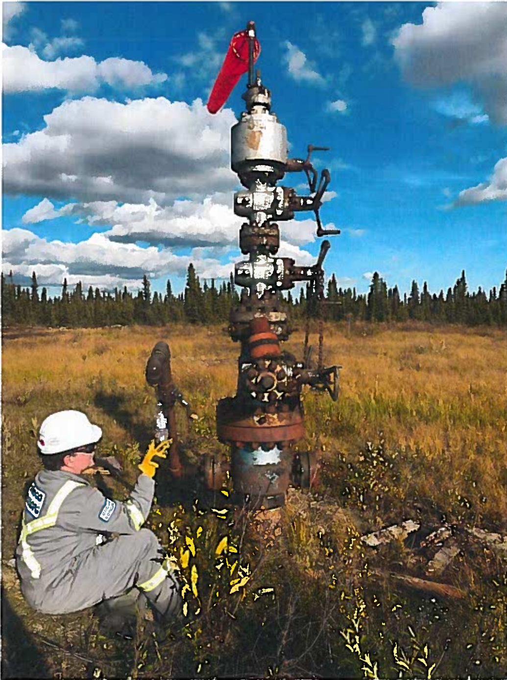
Photo # 1: Well head
