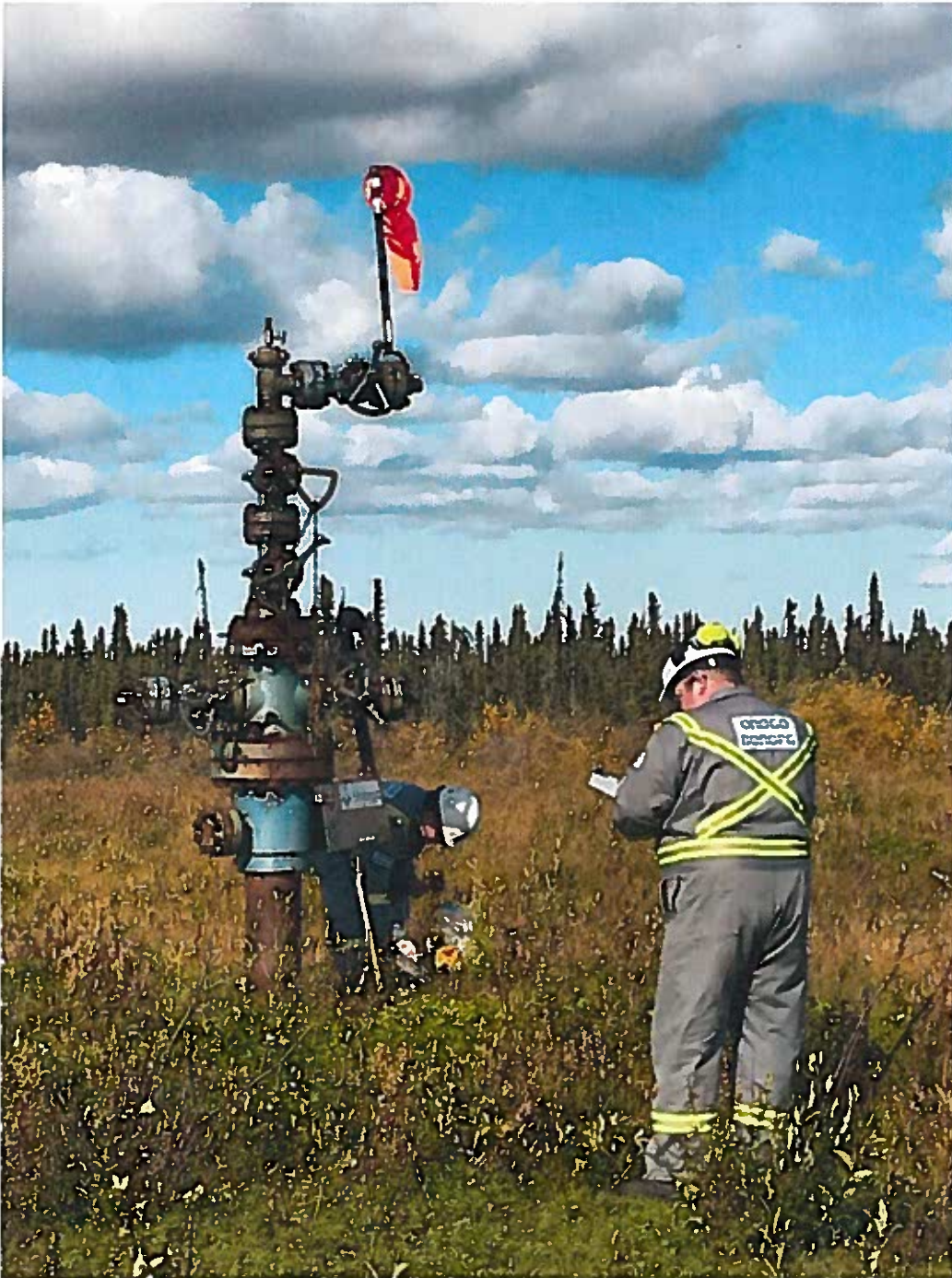
Photo # 1: Well Site - Three well head valves were not secured. All well head valves should be secured to prevent unauthorized operation.
