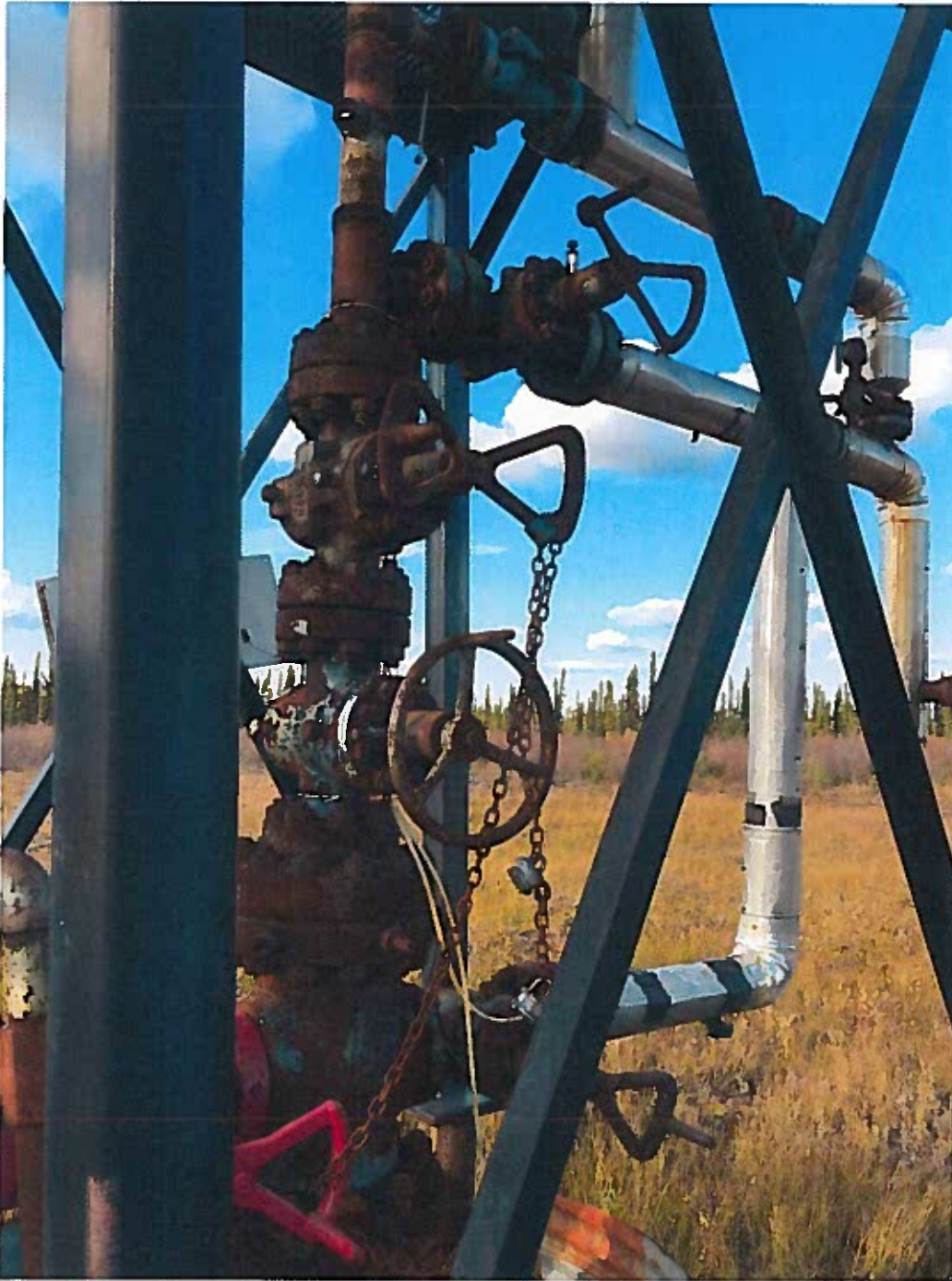
Photo #2: One well head valve not secured. All well head valves must be secured to prevent unauthorized operation
