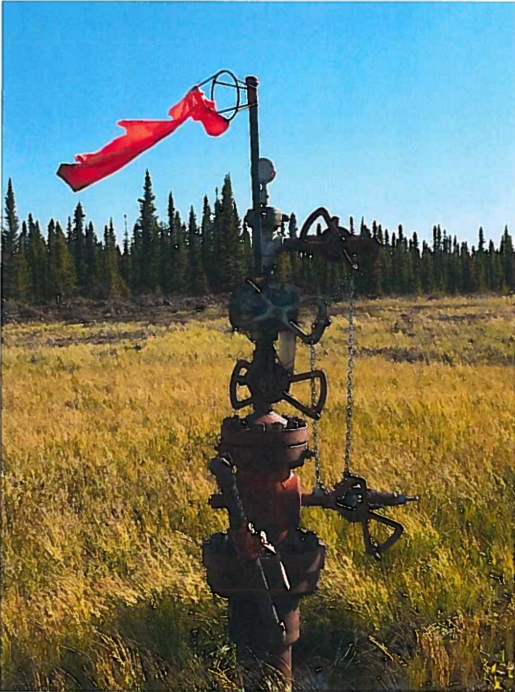
Photo # 1: Well Site - Wind indicator requires repair
