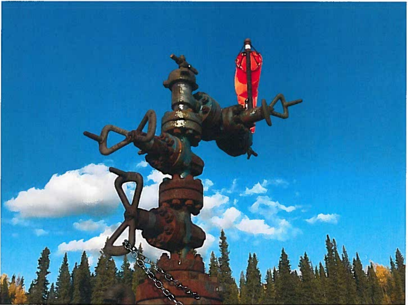
Photo # 1: Well head - Well head valves not secured. Chain too short. All well head valves must be secured to prevent unauthorized access.
