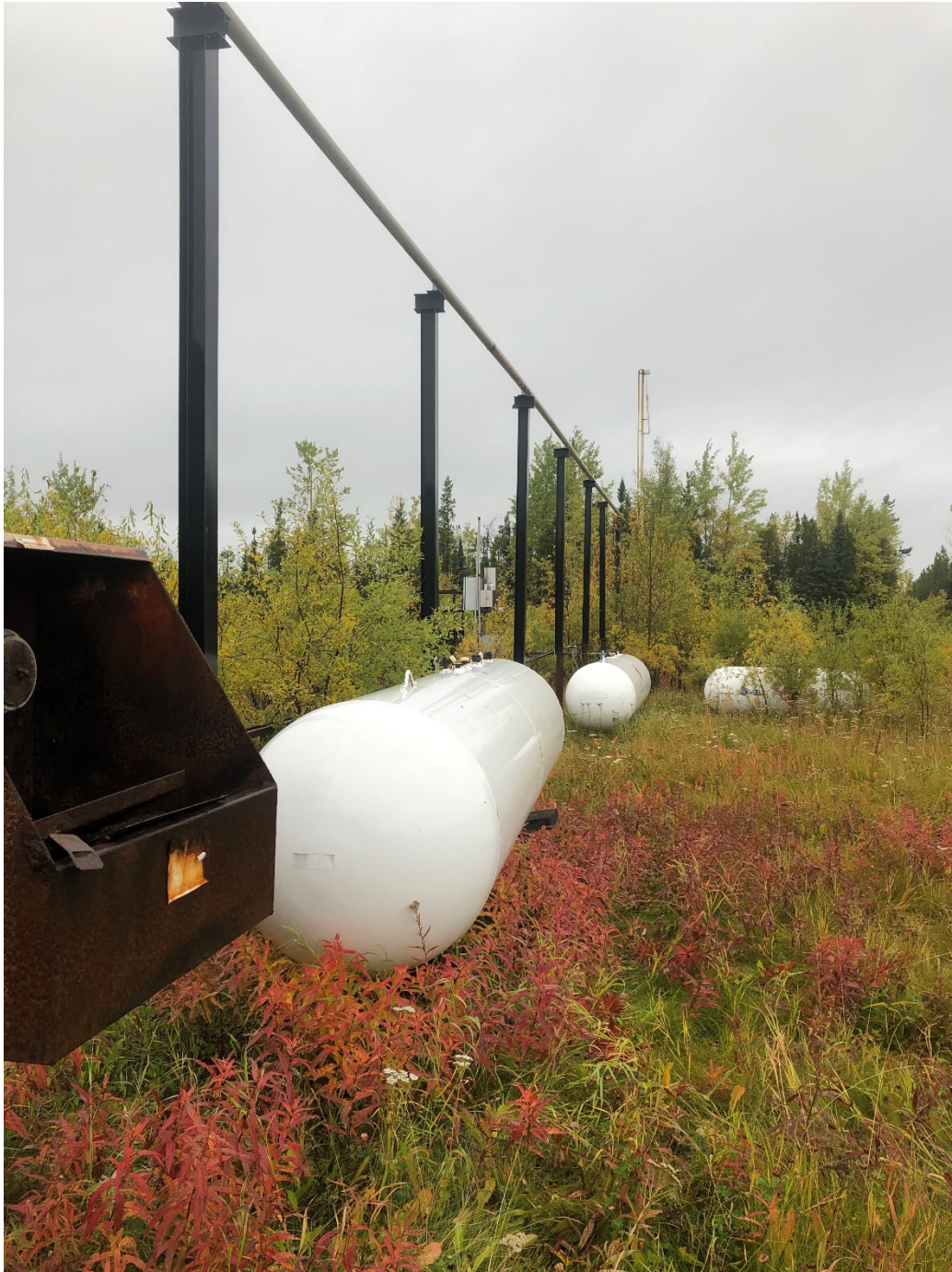
Photo #2: Four (4) propane vessels on site
