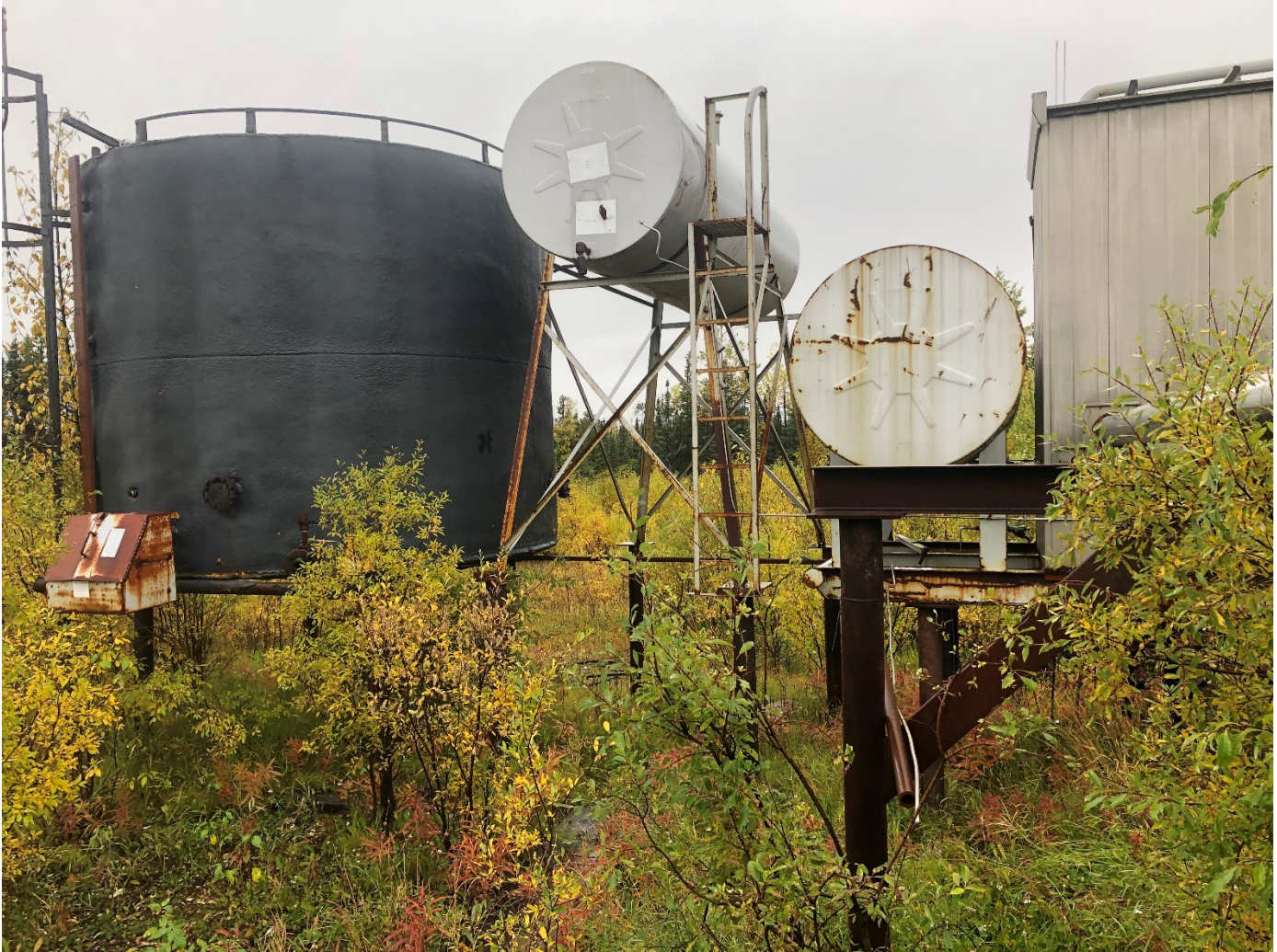
Photo #4: Steel tank directly adjacent the separator building that appears to contain fluid.
