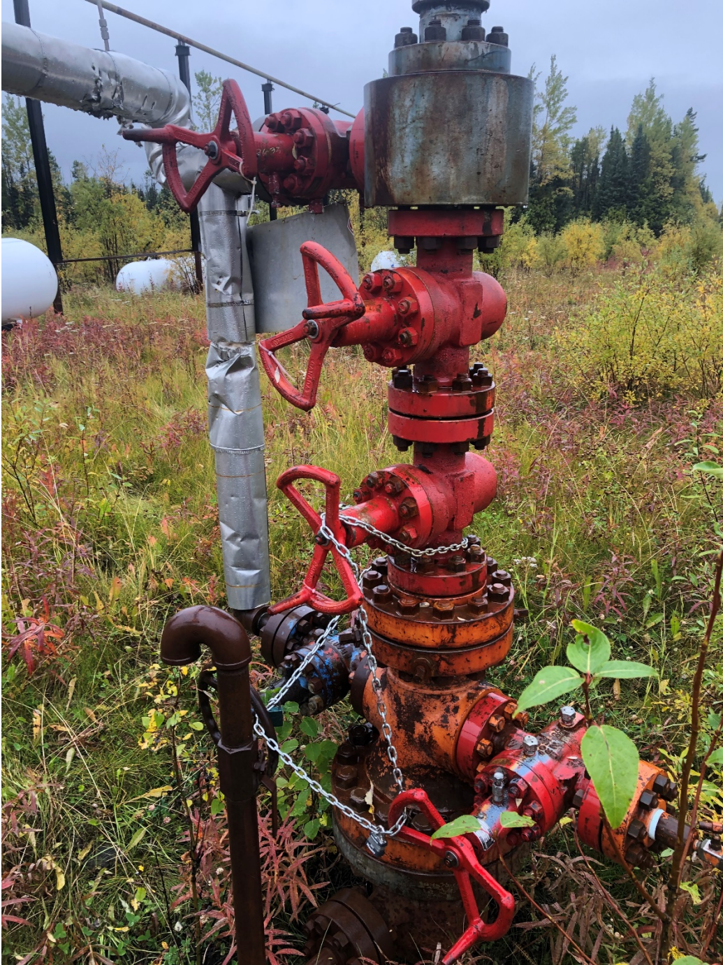
Photo #5: A-73 Wellhead
