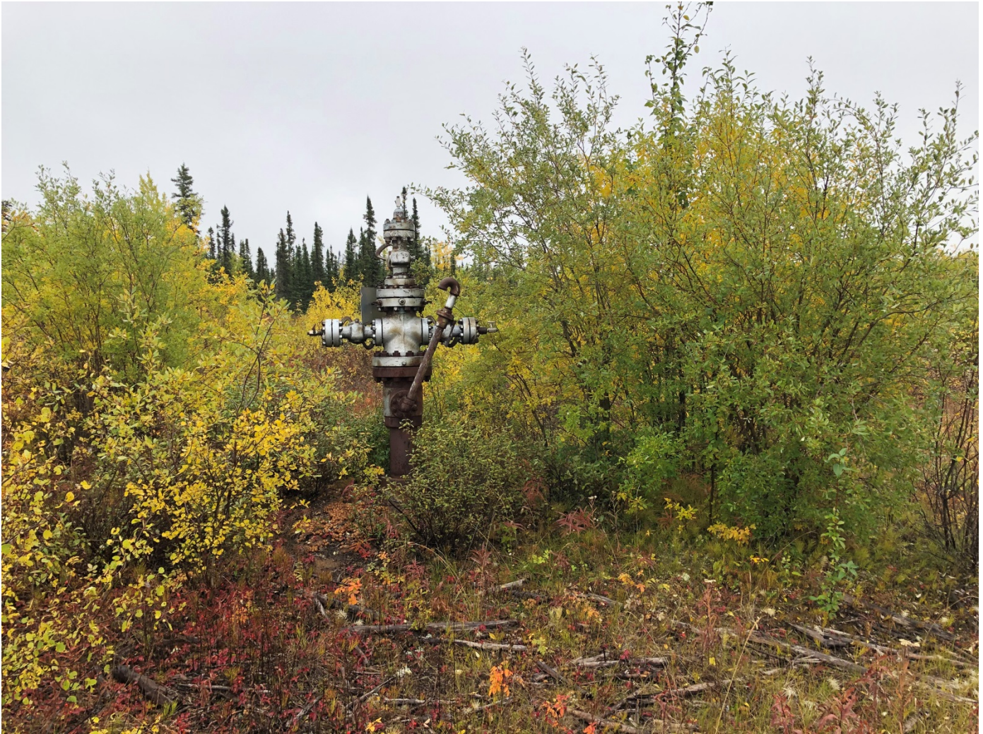
Photo #2: Brush growth adjacent to the well head. All brush must be cleared 10m around the well head. No wind indicator on well site. Wind indicator should be installed on well site.
