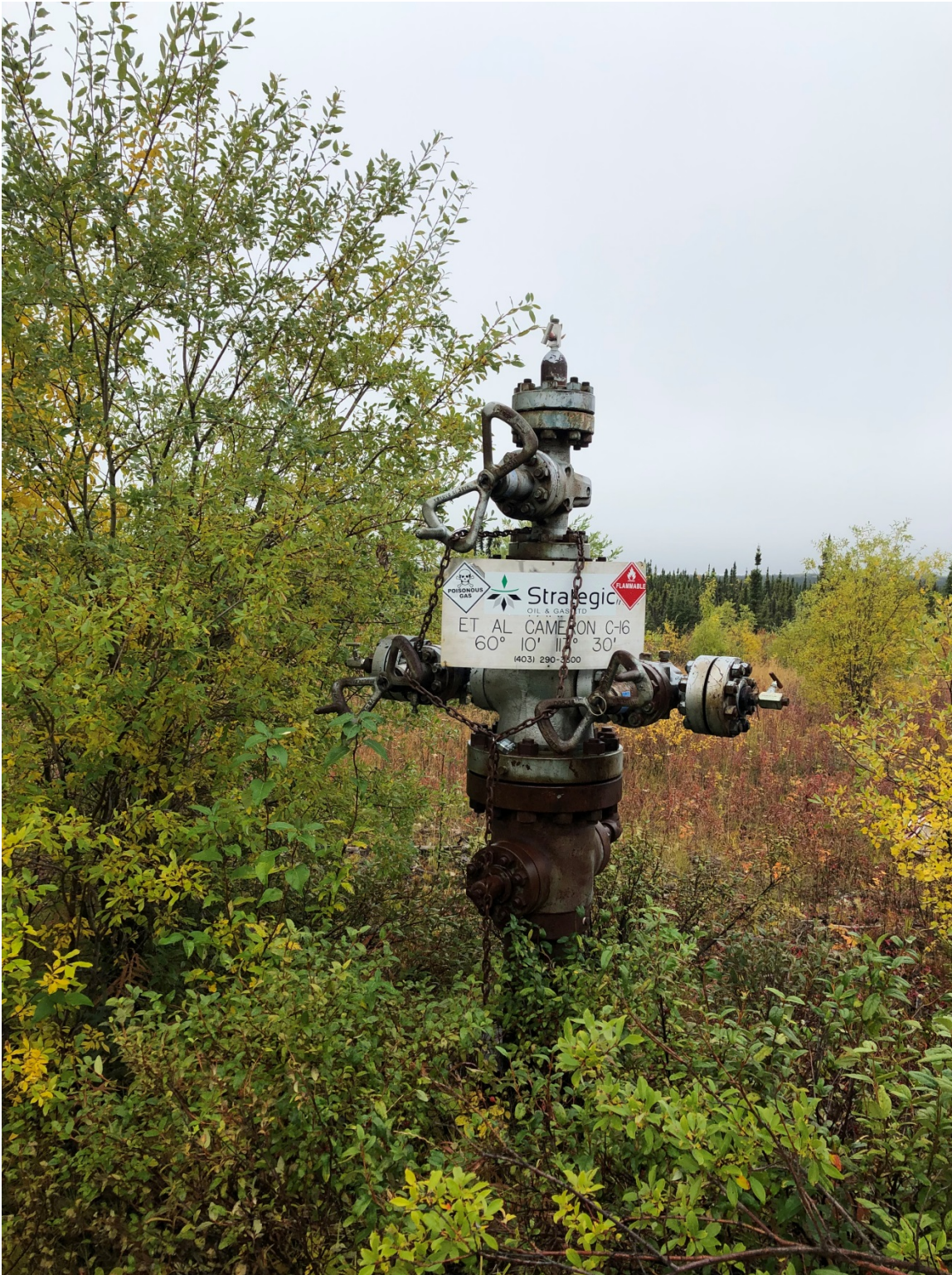
Photo #3: Incorrect 24hr emergency contact number on well sign. .
