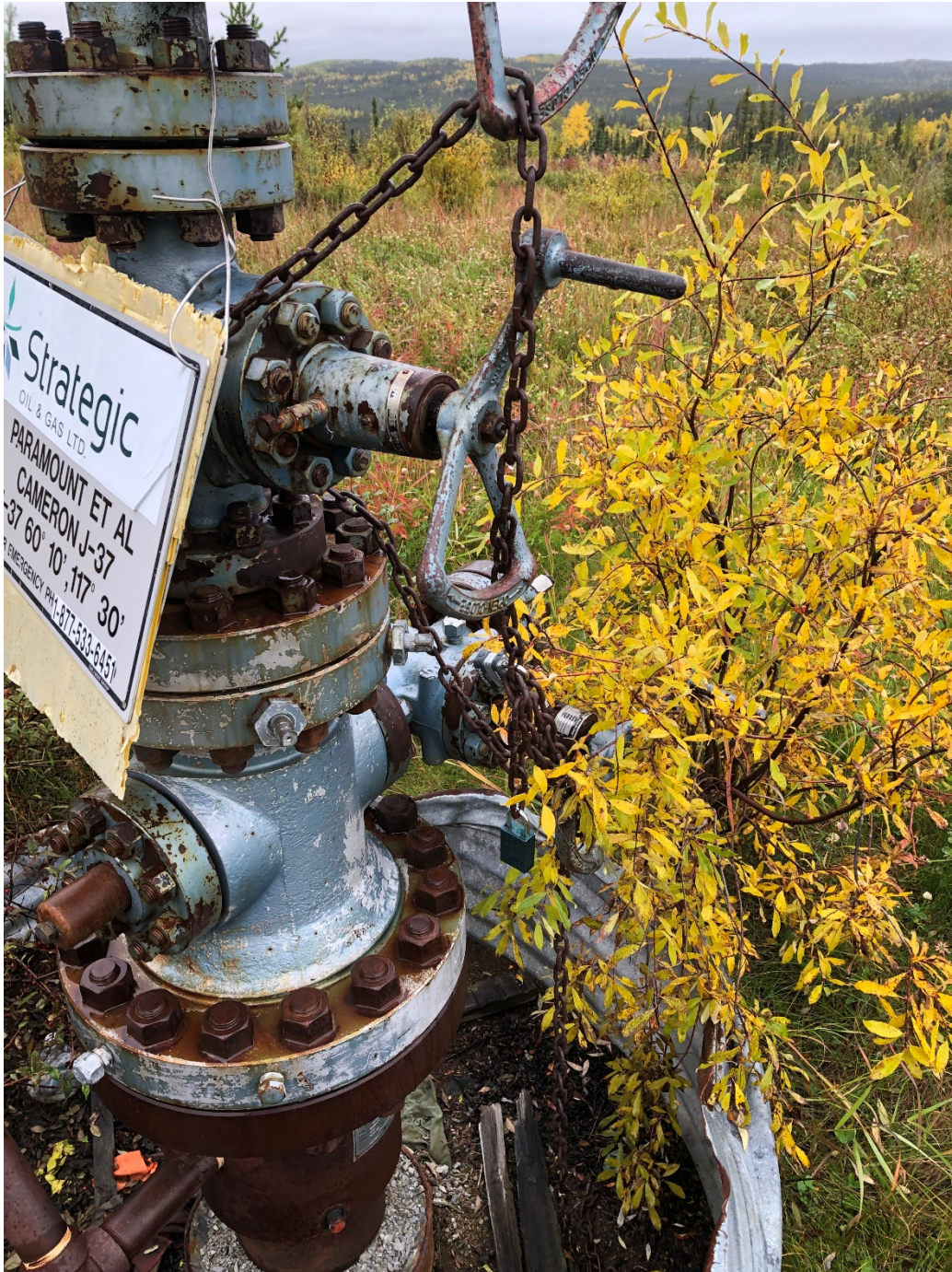
Photo # 2: J-37 Wellhead chained and locked with sign in place
