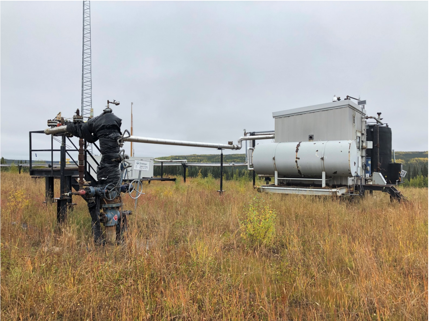
Photo #2: Wellhead and production facilities.
