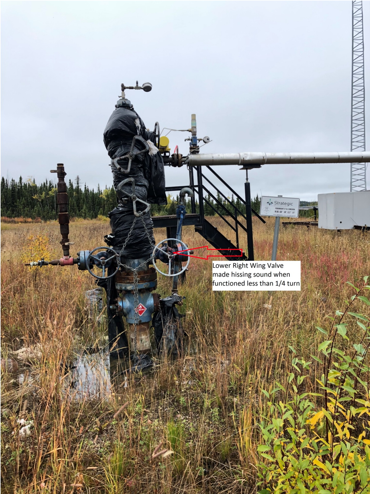
Photo #1: N-06 wellhead - lower right valve.
