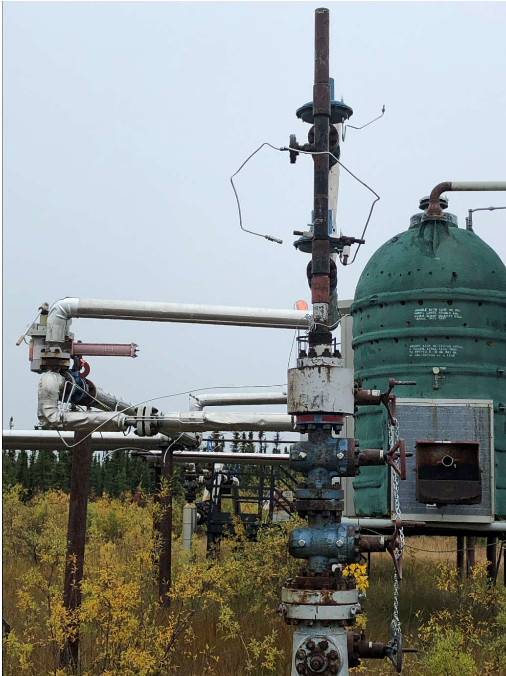
Photo #2: N/28 Wellhead with no well identification sign.
