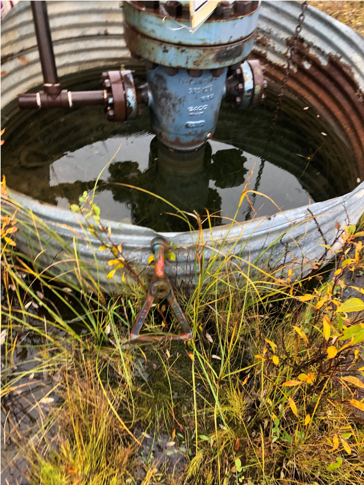
Photo #2: Detached valve handles left on ground and in conductor hole.
