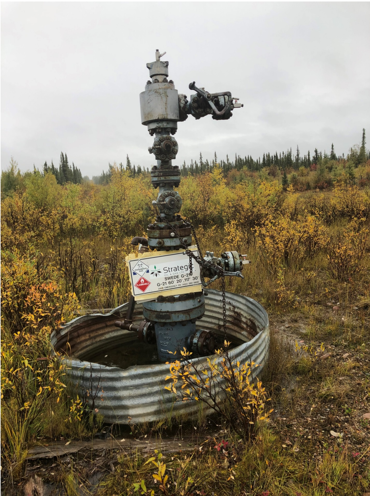
Photo #: No wind indicator on well site. Wind indicator should be installed on well site. All well head valves should be secured to prevent unauthorized operation.
