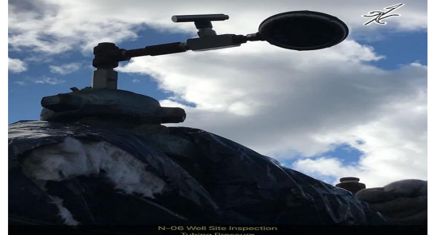
N-06 Well Site Inspection Tubing Pressure
