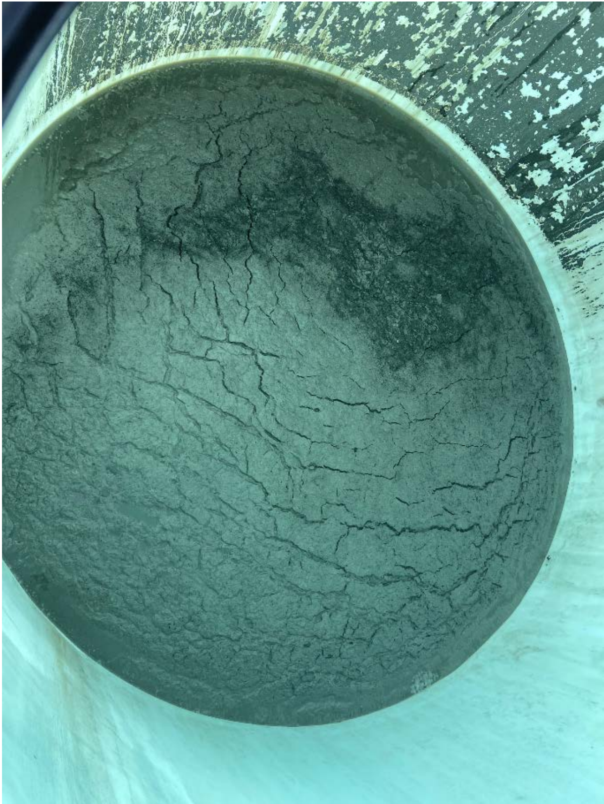
Figure 12 - L-68 SCVF catch tank inside - 2021-04-29
