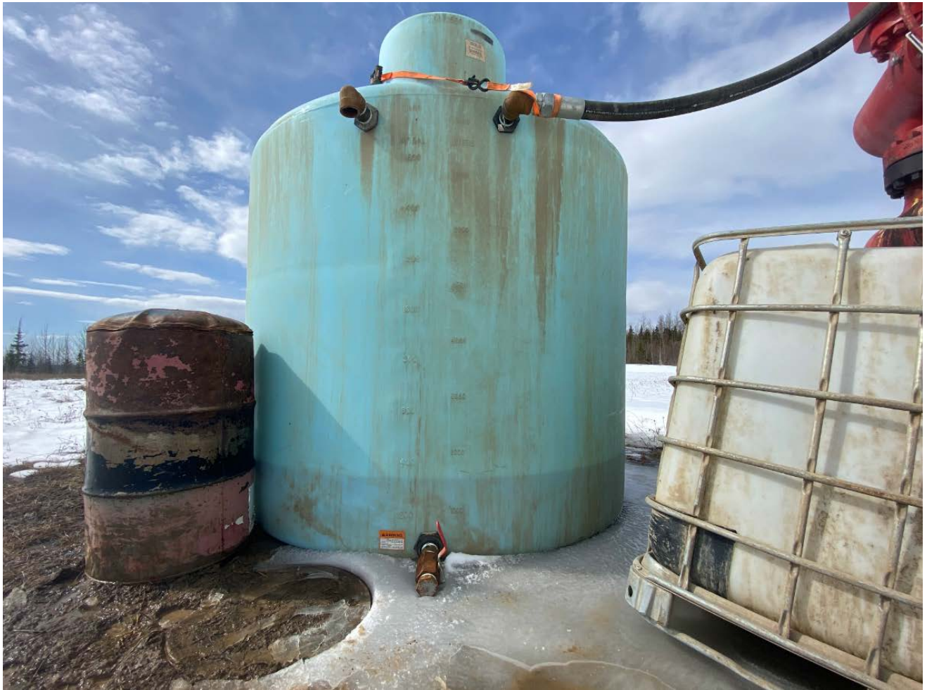
Figure 10 - L-68 SCVF catch tank - 2021-04-29
