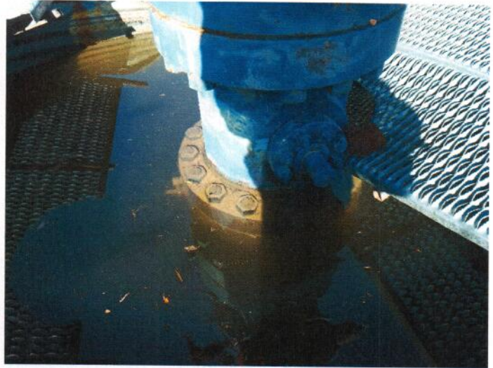
SCV not visible and grating displaced in 2020
