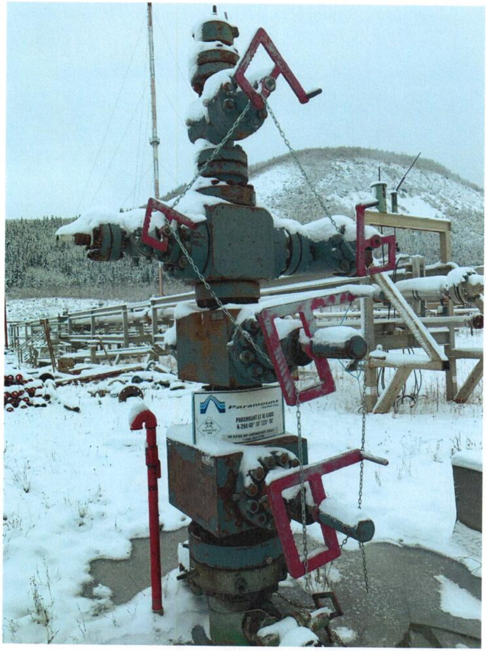
K-29A Wellhead October 14, 2020
